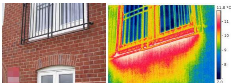
Photograph and thermal image of Juliet balcony
