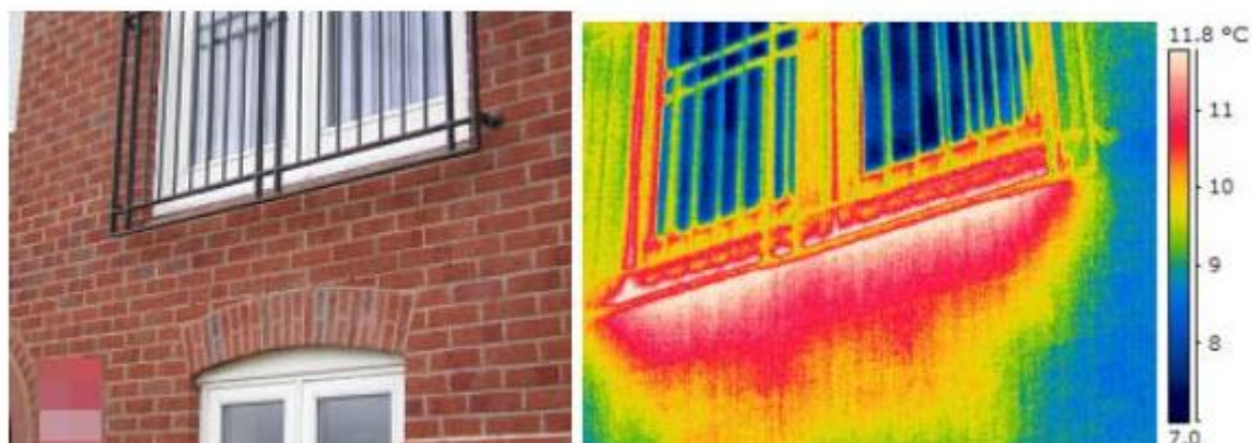
Photograph and thermal image of Juliet balcony
